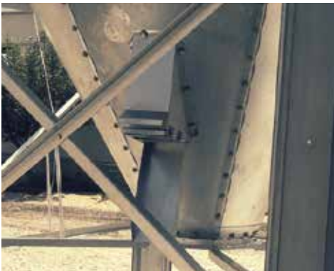
AUXILIARY NOZZLE IN HOPPER
