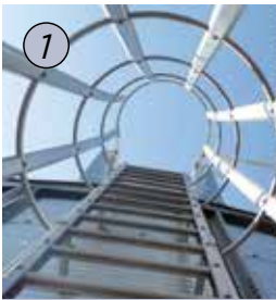
1 LADDER TO ROOF
